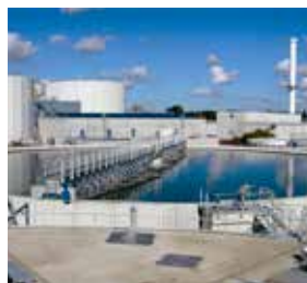
Waste water treatment
